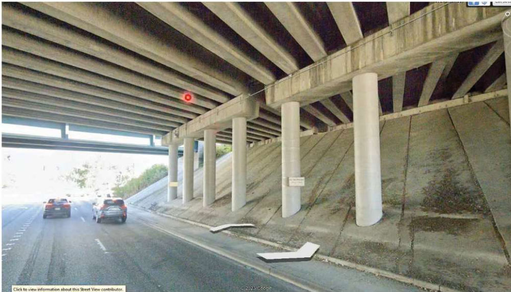
I-405 MAIN LINE BRIDGE OVER TALBOT ROAD STREET VIEW FROM GOOGLE EARTH (LOOKING WEST)
